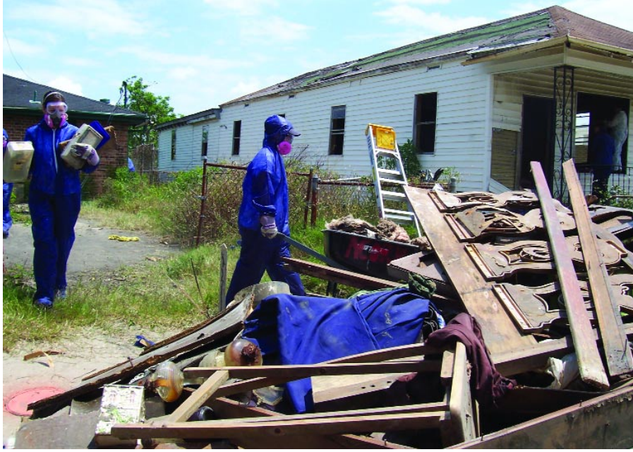
Nearly two years after the storm, debris from homes in the lower ninth ward, one of the hardest hit parishes in New Orleans, is still being removed with the help of local organizations and volunteers from across the nation.
