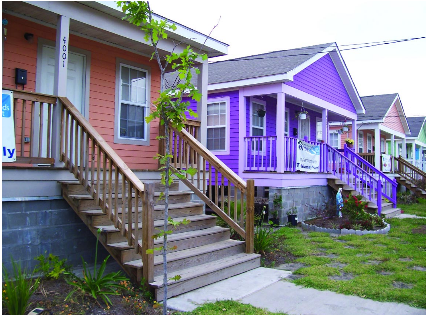
Single-family homes go up in the upper ninth ward to bring back residents displaced by Katrina.
